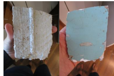
Plaster found behind the existing wall material
