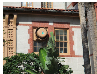
Existing Mechanical Equipment
