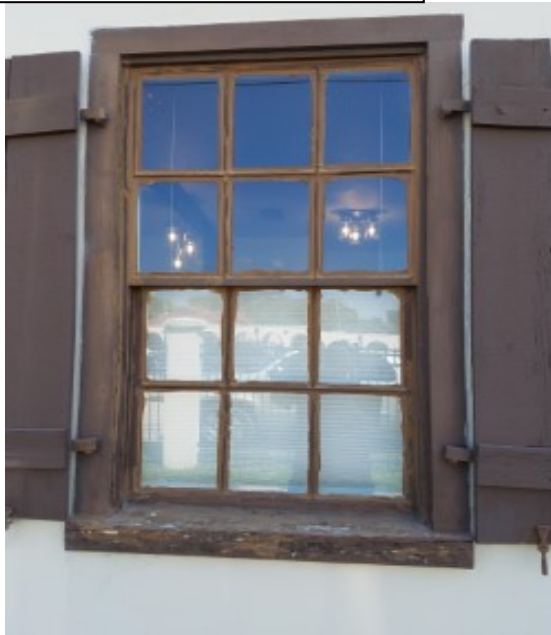
West side of home facing Charlotte St. This side has the most significant damage.
