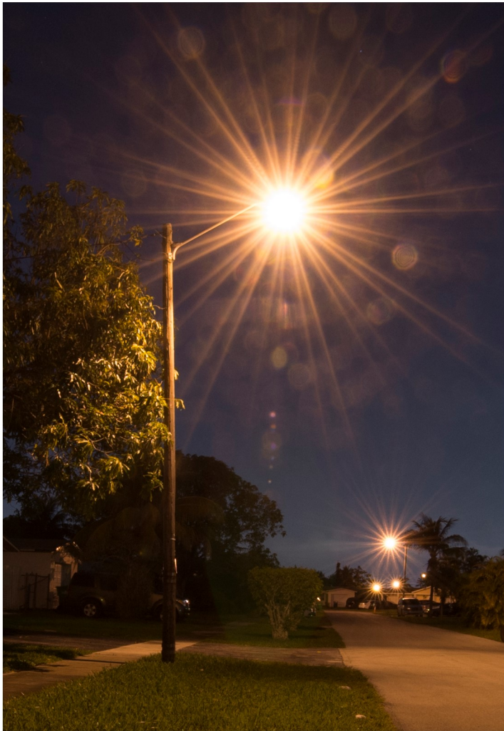
Existing 2200 Kelvin HPS
