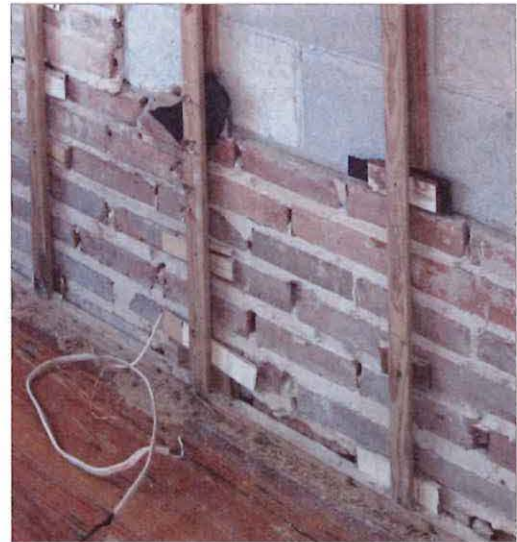
Although the brick may be an acceptable flood resistant material, the lack of mortar provides a path for flood water ingress. (Photograph courtesy of the City of St. Augustine.)
