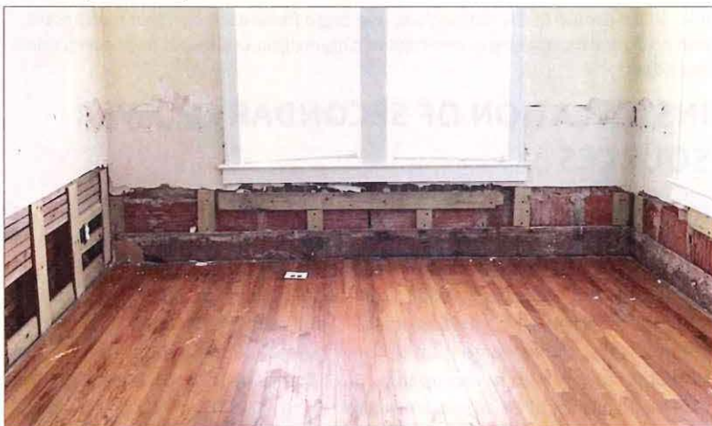
Lower portion of wall finish removed in Lincolnville home to allow the cavity to dry out following a flood revealing sub-standard work from prior recovery effort. Electrical service should be elevated if home remains at current elevation. It is always prudent to use licensed contractors. (Photograph courtesy of the City of St. Augustine.)
