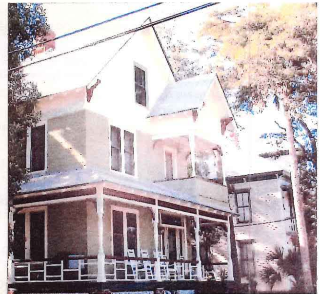
The siding on this building was altered (ca. 1930-50s) and shows the impact of replacement finishes that change the scale and detail of the building's historic character. Restoring the Queen Anne siding would be a staff-approvable request. Also note for reference the scale of historic horizontal siding shown on the adjacent historic building.
