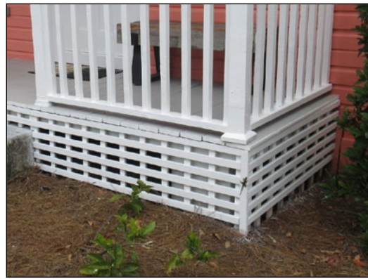
Do not use foundation screening in such a way that it entirely obscures structural piers.
