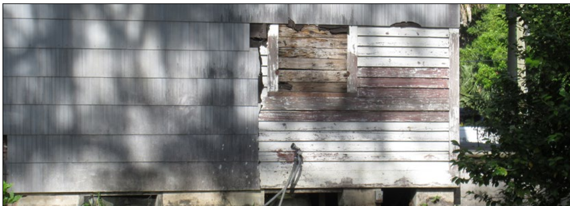
Missing asbestos singles reveal the historic wood siding underneath, as well as the outline of a window that has been infilled.
