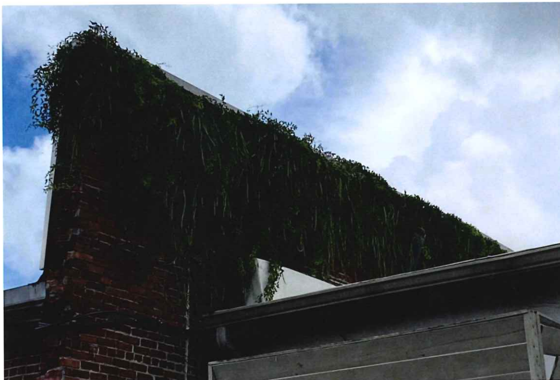
Photo 1.03 - Wall at alley (Spanish Street) showing cant, missing mortar, and vegetation
