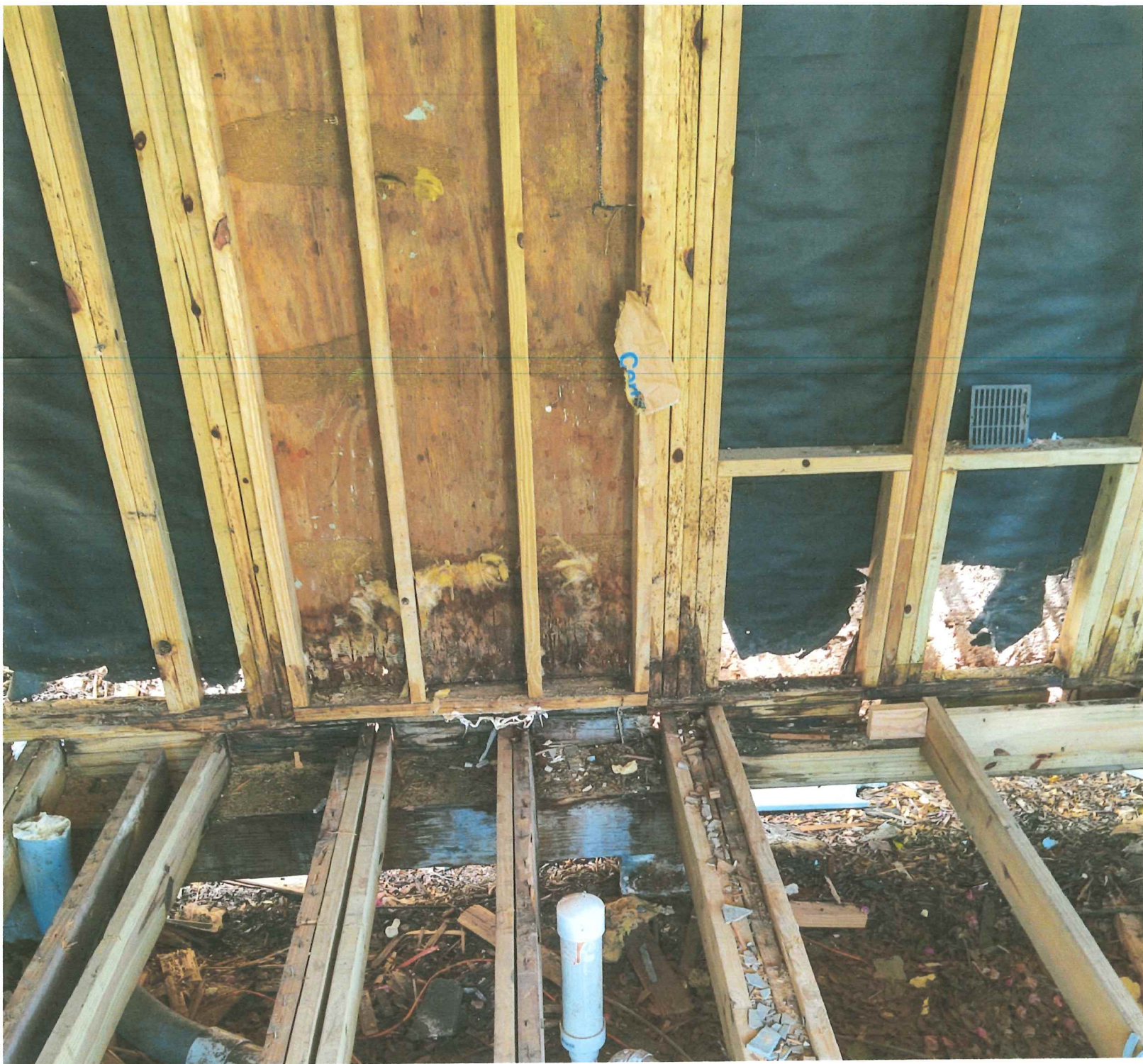
ROTTEN SILL BEAM
