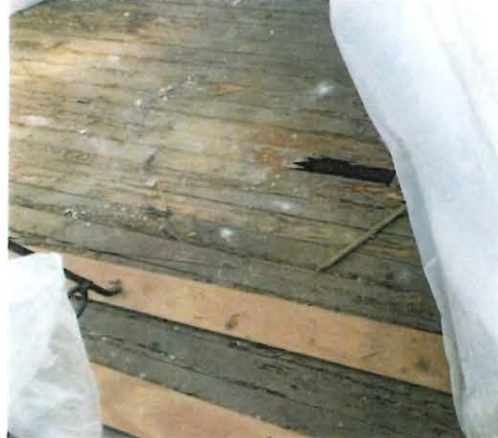
Image 7: Termite Infestation Evidence
