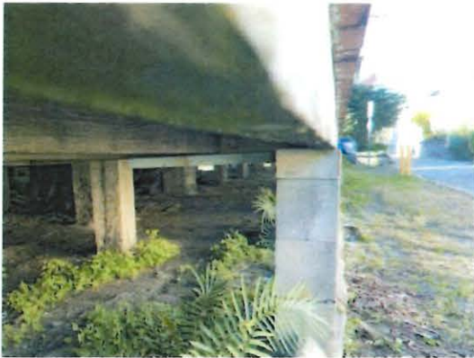
Image 1: Out of Plumb Pier
