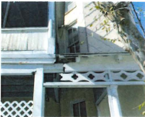
Image 9: Wood Beam Failure
