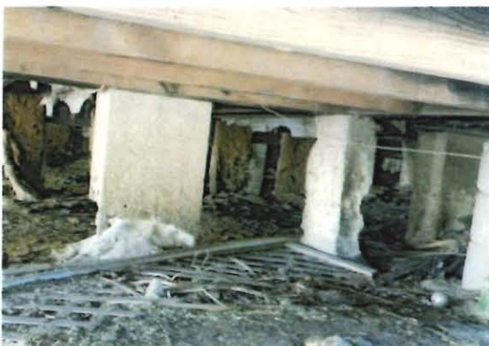
Image 3: Visible Section Loss to Piers
