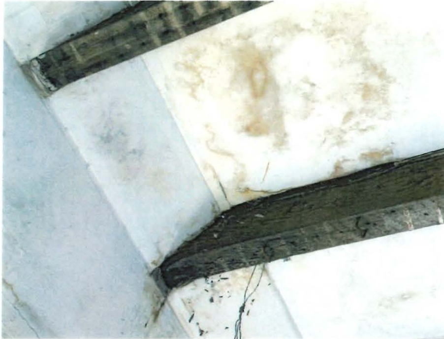
Image 8: Joists with Moisture Rot
