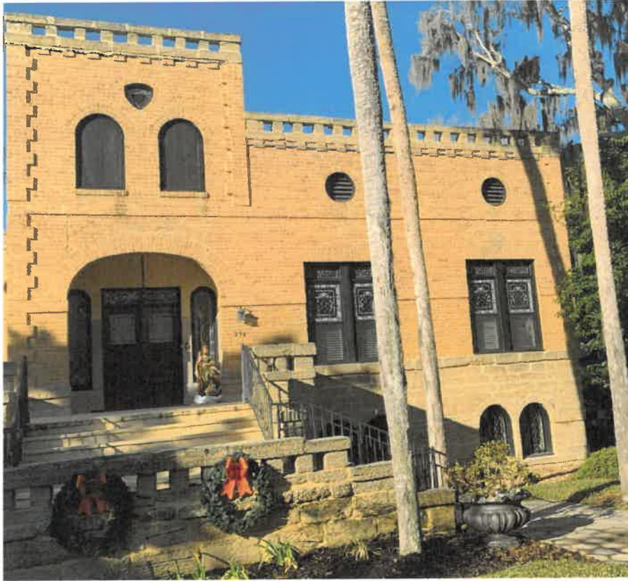
Figure 6. East wall, lower portion repaired in 2017, no work done on upper wall.
