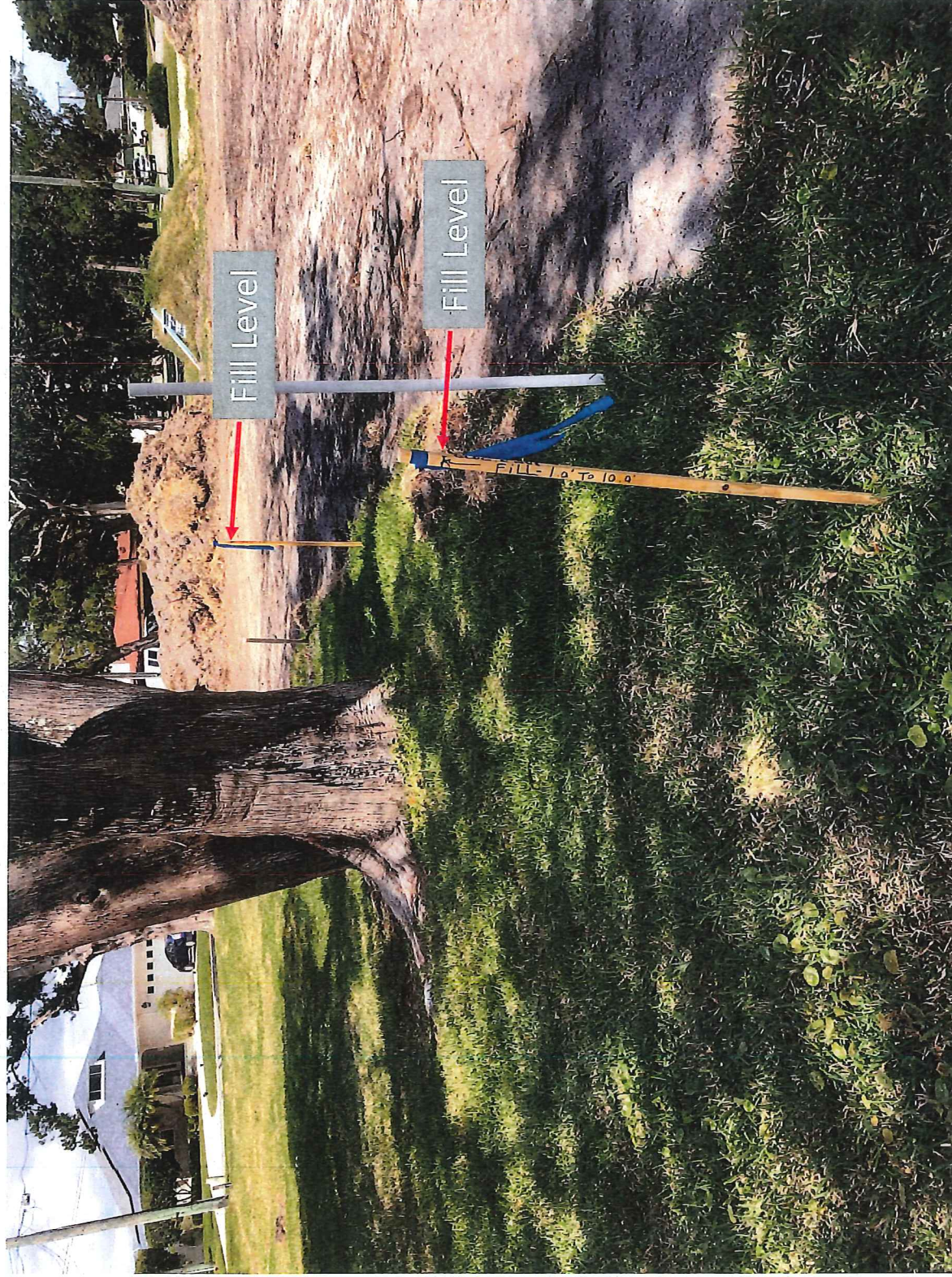
Figure 7 – Lot Grading Fill Impacting Protected Trees
