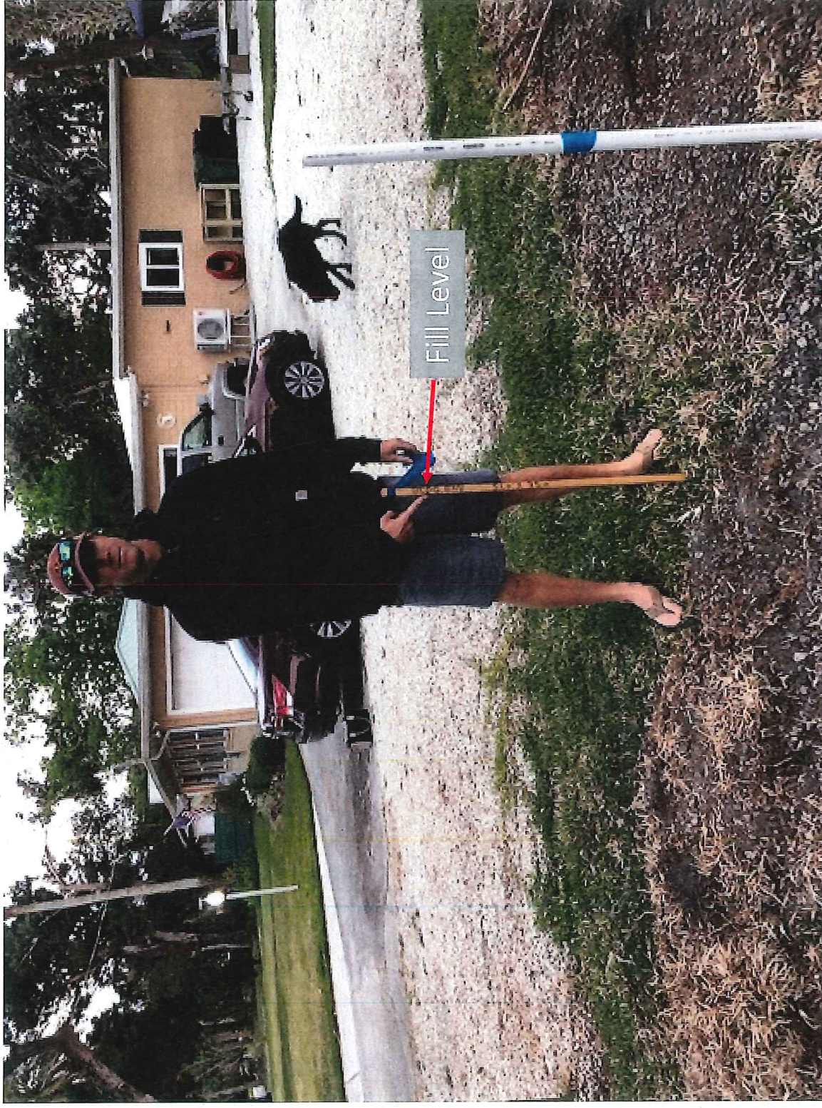
Figure 6 – Lot Grading Fill Issue – 7.5 Ft from Property Boundary
