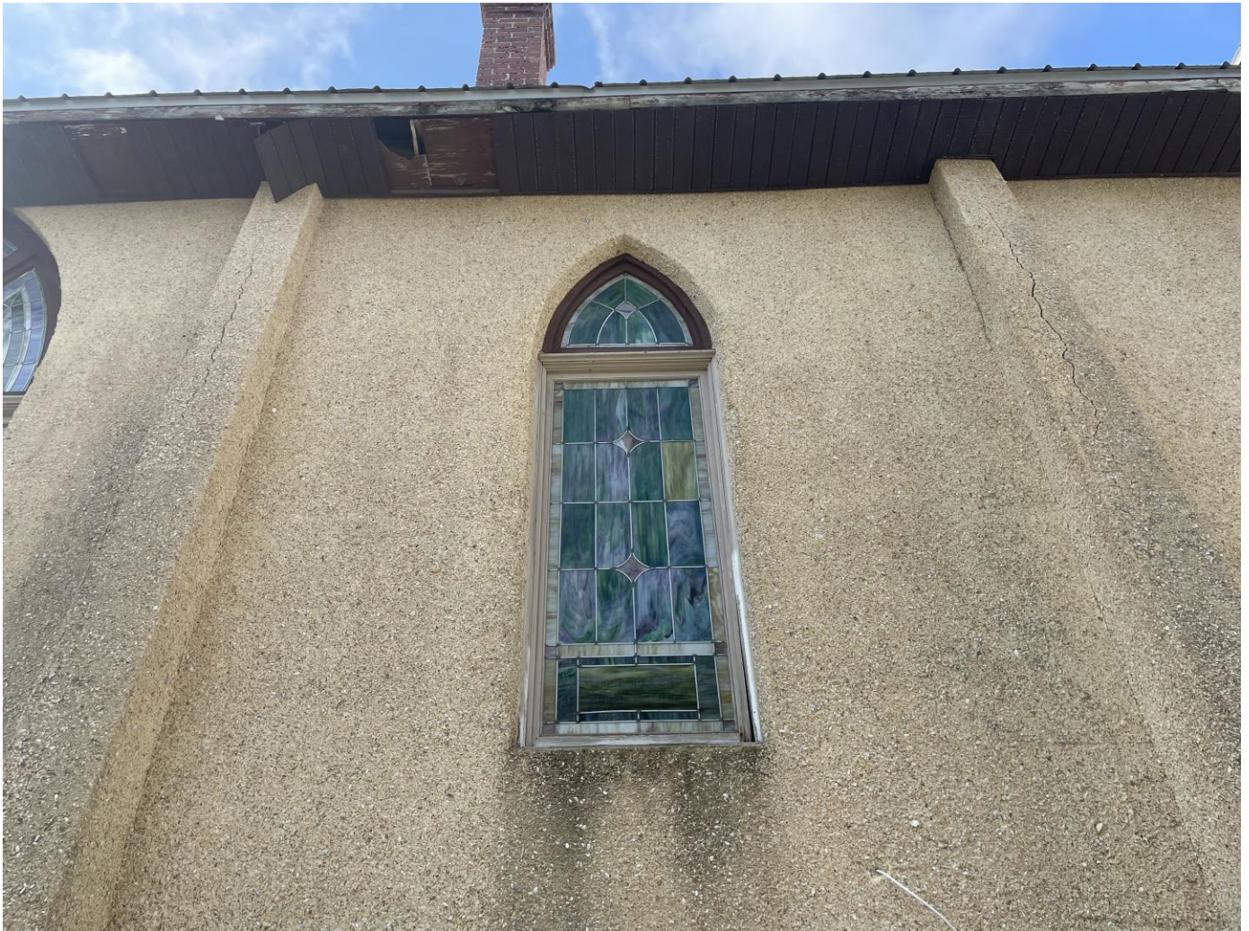
Window to be restored.
