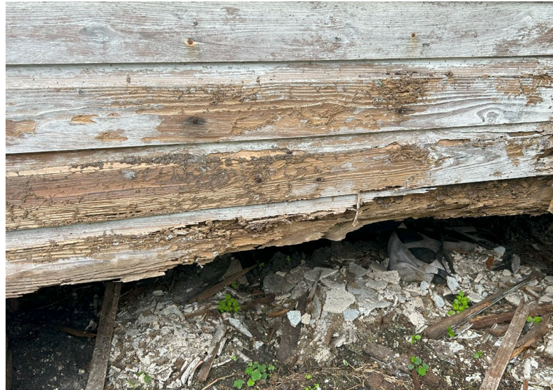
Examples of Deterioration (no specific order)
