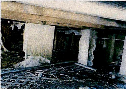
Image 3: Visible Section Loss to Piers
