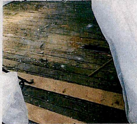
Image 7: Termite Infestation Evidence
