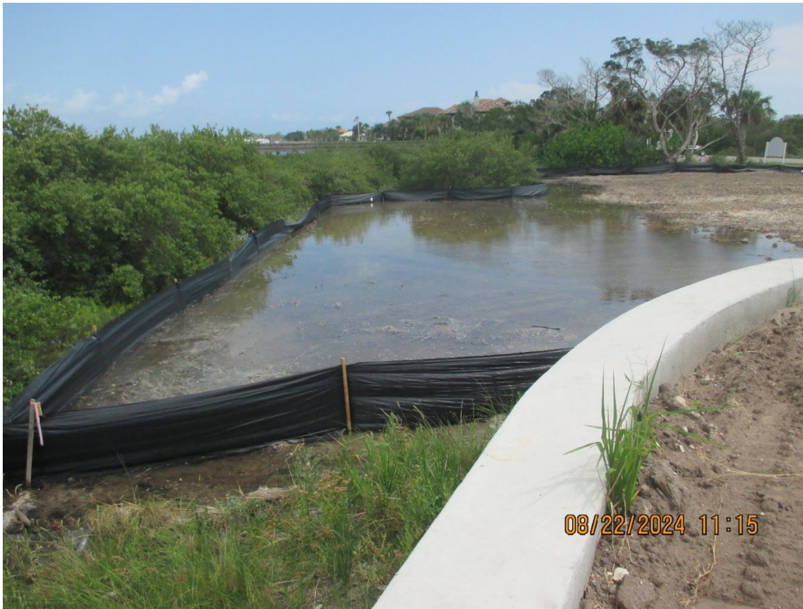
Figure 4- Current erosion control measures.
