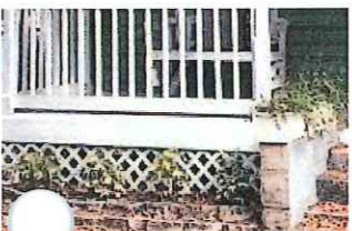
Example of Raised Pier construction with porous skirting (lattice). Image from ML+H.
