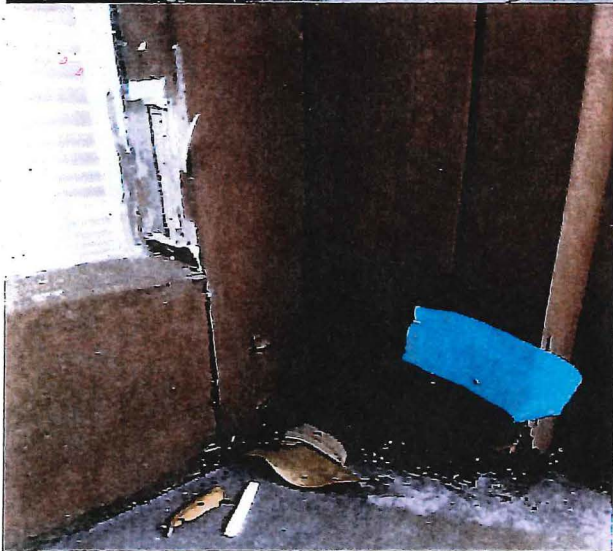
South facing portion of home, not seen from road, windows face neighbor's house. Both windows have significant damage.
