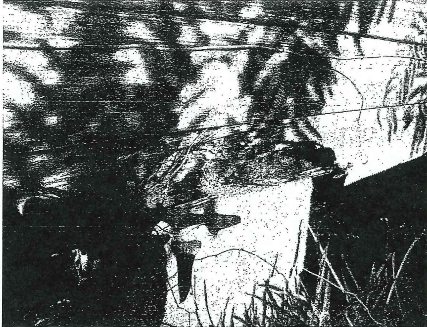
Picture 5 – Insect Damage at Beam Bearing Location
