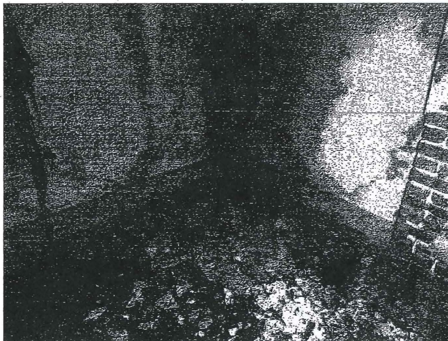
Picture 15 – Damaged Interior Finishes/ Water Damage
