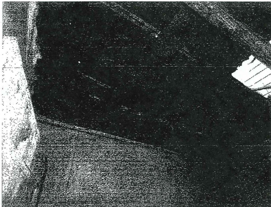
Picture 1 – Deteriorated Metal Roof and Roof Leak
