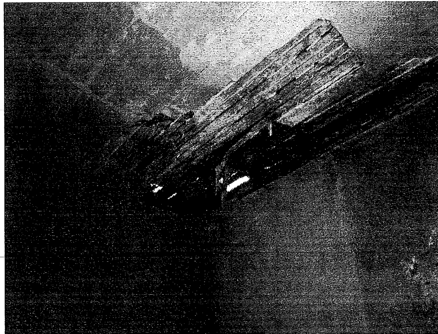
Picture 2 – Roof Leak
