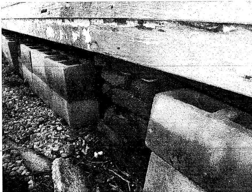
Picture 12 – Deteriorated Brick Pier
