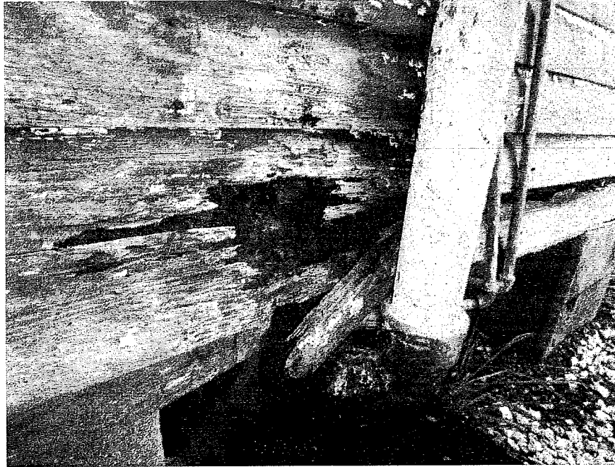
Picture 11 – Damaged Siding
