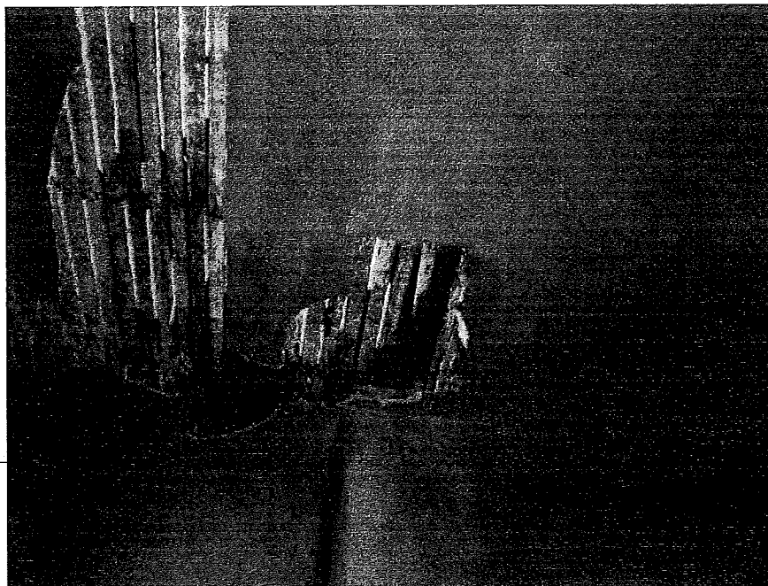
Picture 14 – Damaged Plaster
