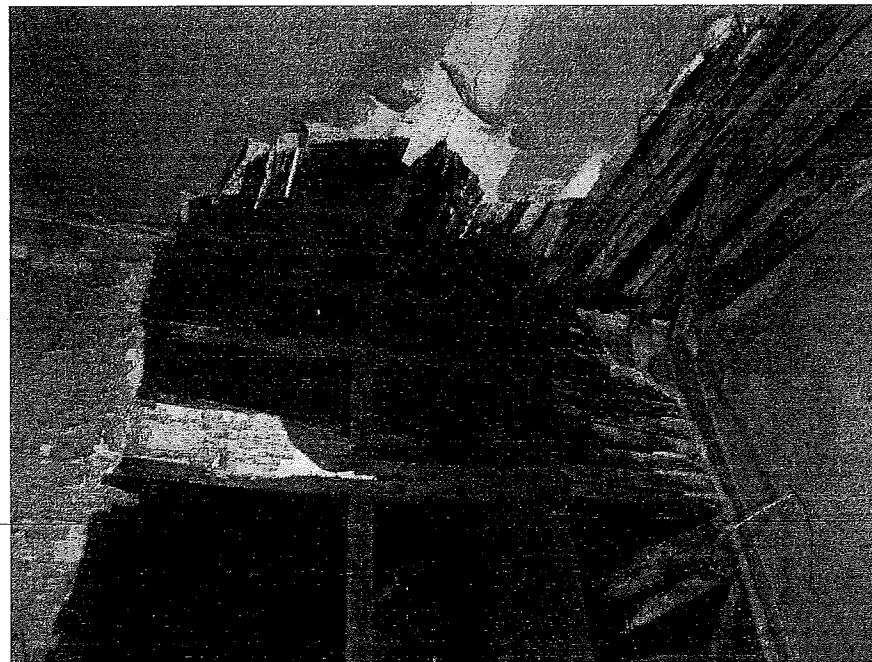
Picture 16 – Damaged Interior Finishes
