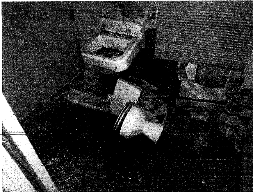
Picture 8 – Collapsed Floor System
