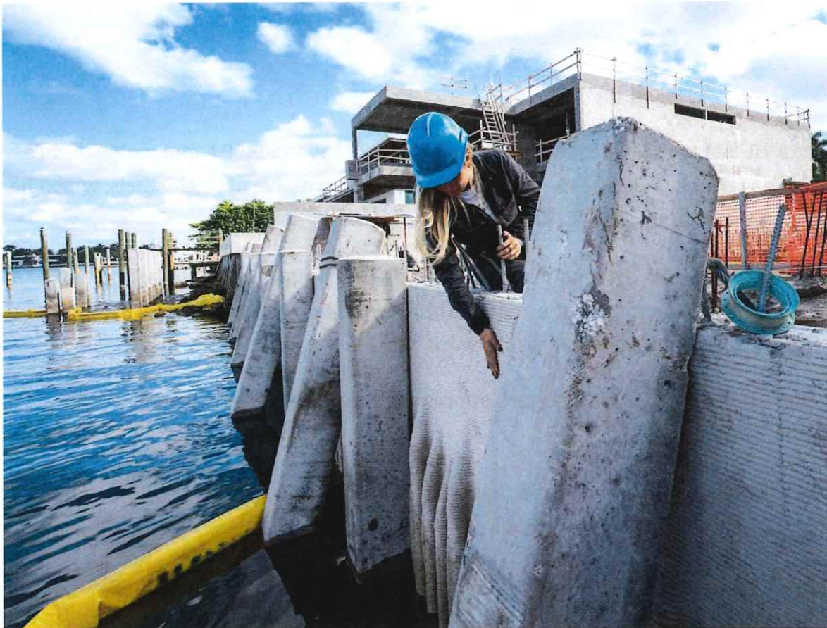
Founder and CEO of Kind Designs, Anya Freeman, inspects a 3D printed seawall in Miami Beach. Sophia Bolivar sophiabolivar@outlook.com
