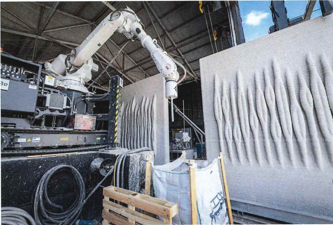
Seawalls at the Kind Design headquarters in Miami are produced using what is billed as the world's fastest concrete 3D printer. Sophia Bolivar sophiabolivar@outlook.com
