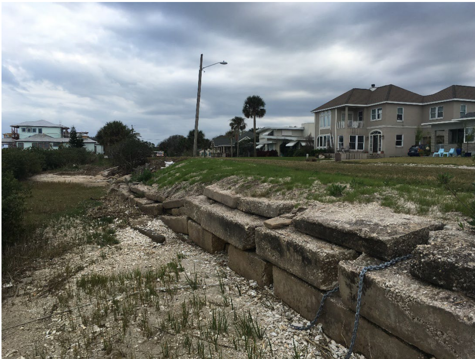
Inlet Drive Shoreline and Existing Coquina Block Wall. Post Hurricane Irma (2017). Facing South.
