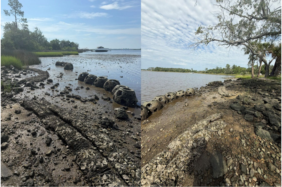
Jacksonville Zoo Living Shoreline Project. Oyster gabions with reef balls. *Photo credit, SWCA Environmental Consultants*
