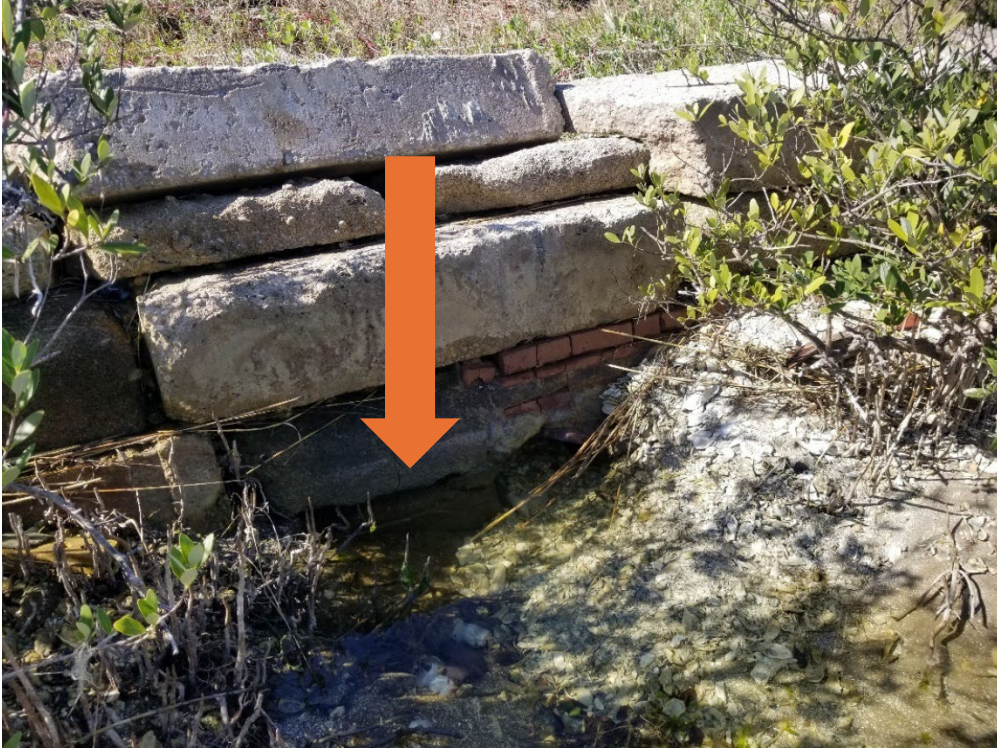
Existing stormwater outfall (clay pipe) to be replaced and reset at a higher elevation as part of this project.
