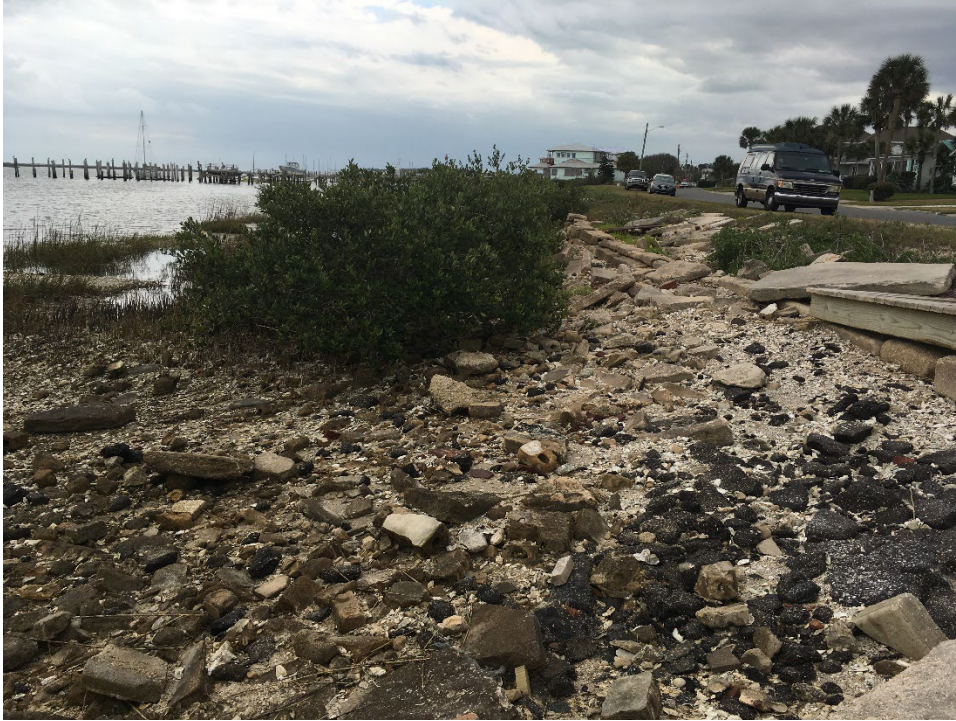
Inlet Drive Shoreline, Post Hurricane Irma (2017). Facing South.
