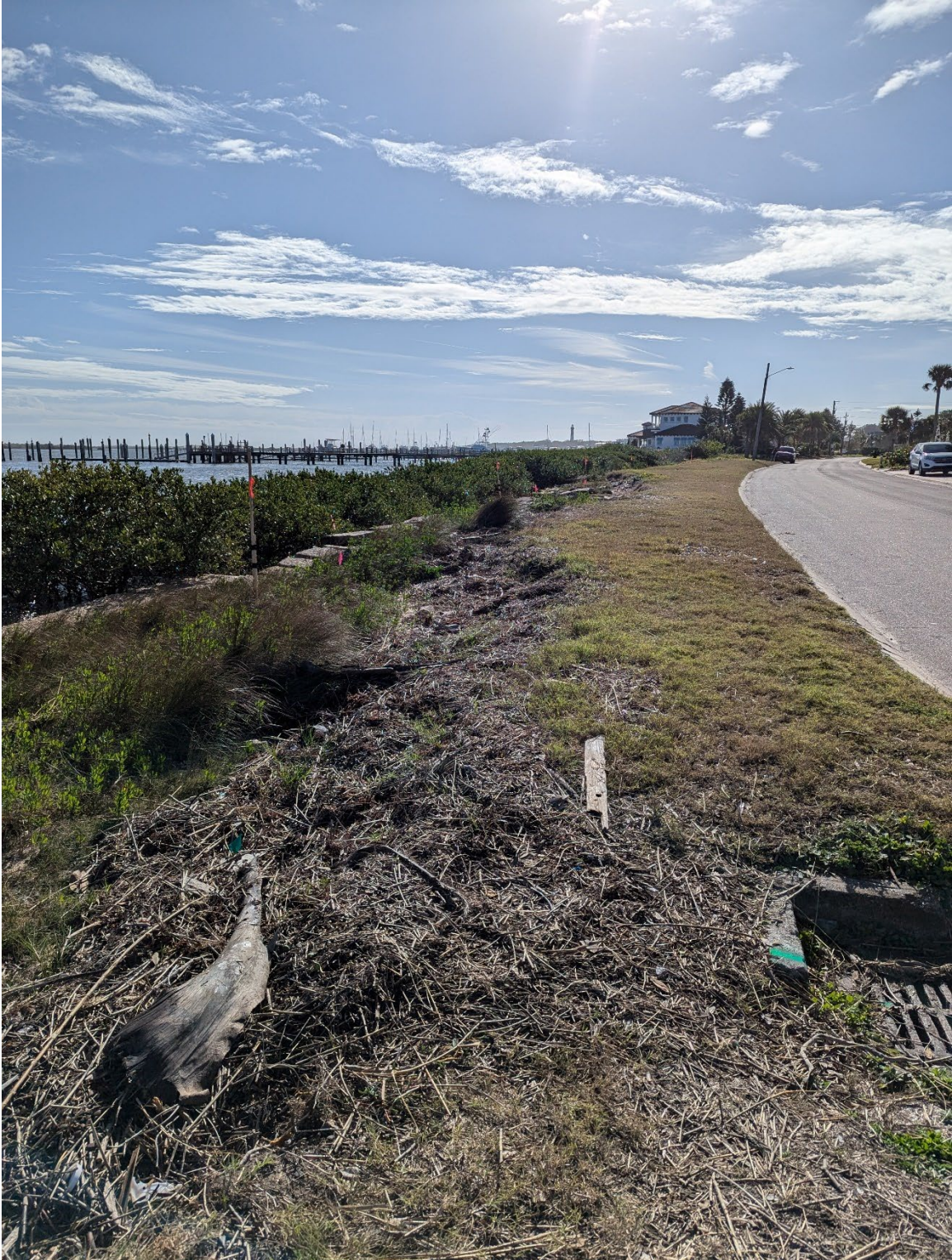
Proposed wall alignment staked by surveyor. Orange flag represents the top of the proposed wall.
