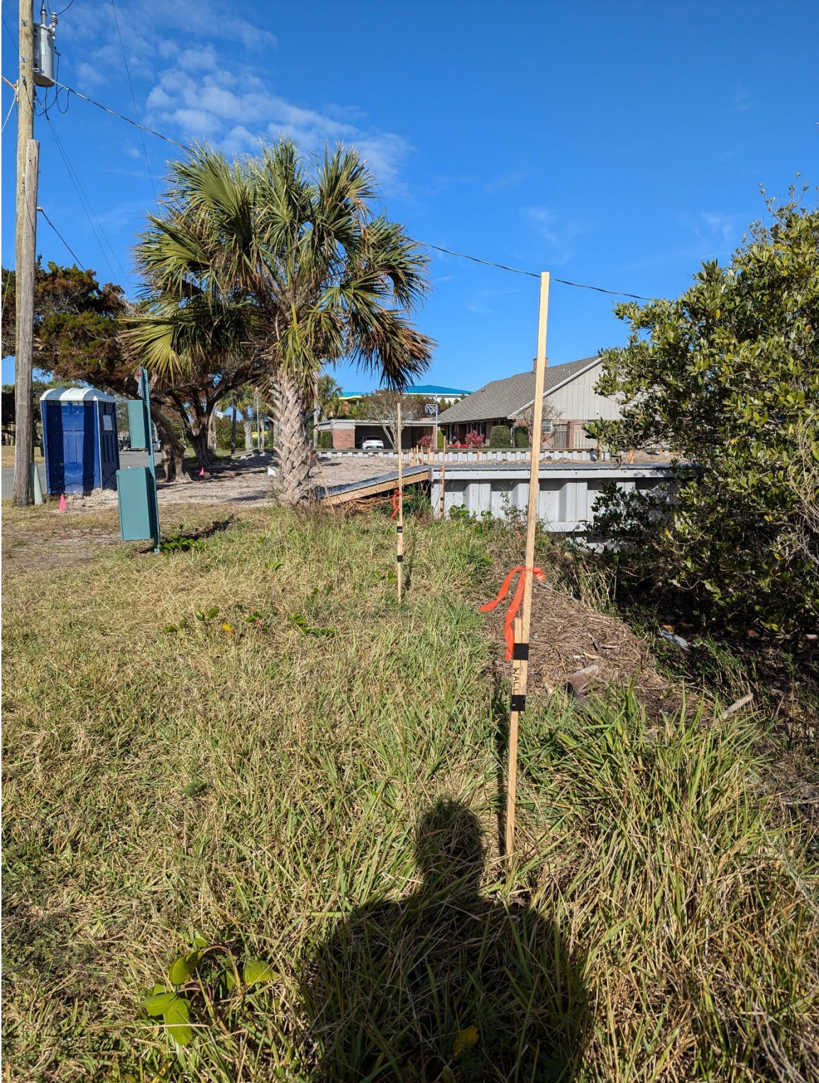
Proposed wall alignment staked by surveyor. Orange flag represents the top of the proposed wall.
