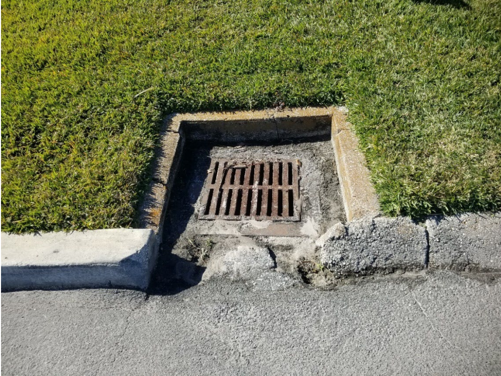
Existing stormwater inlet (one of two) that will be replaced as part of this project.
