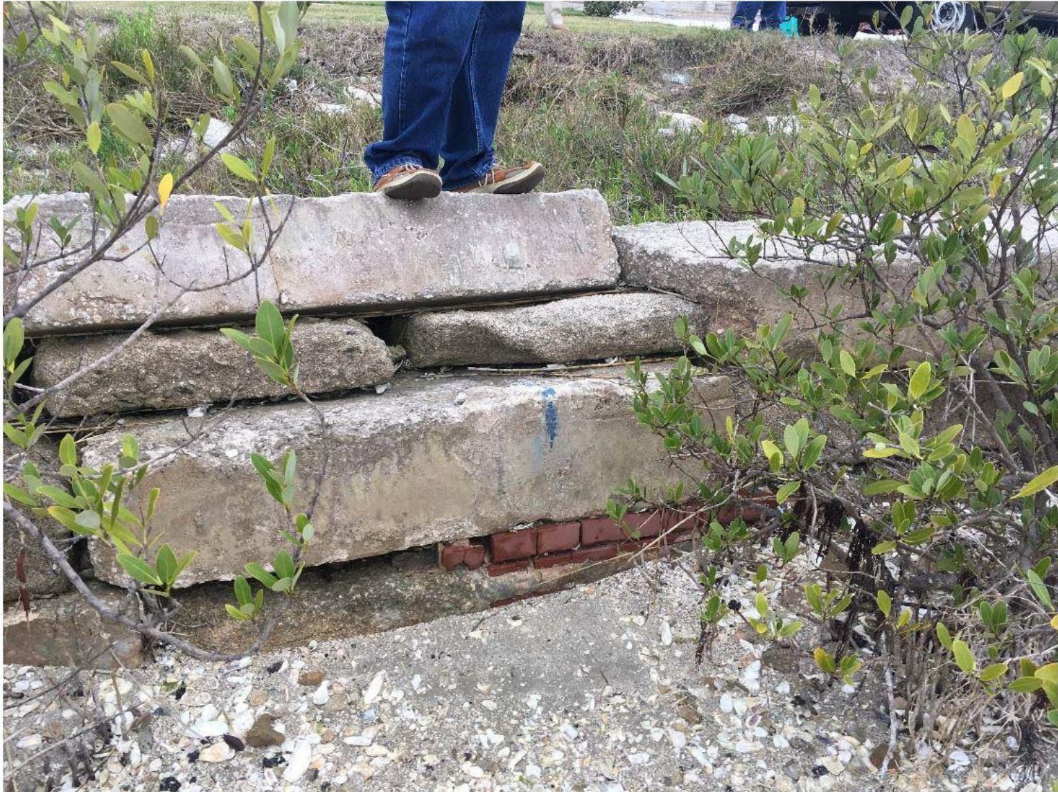
Figure 2 - Stacked masonry showing no mortar and a partial layer of used bricks, view to west
