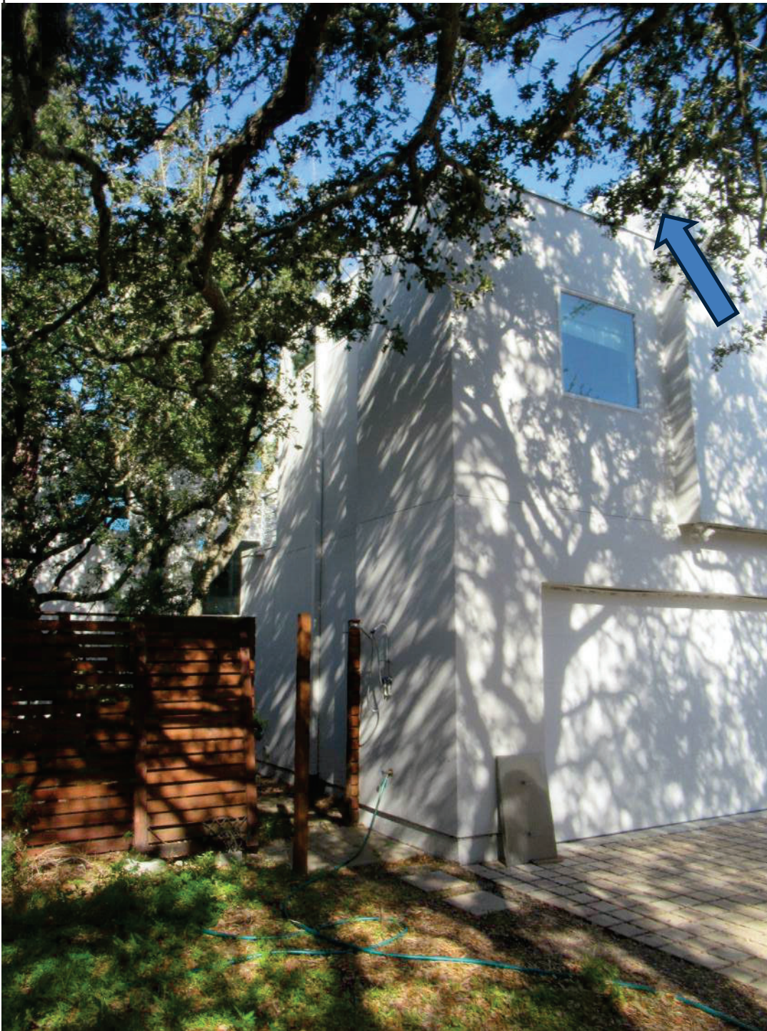
Photo of existing 3 rd story roof deck at southwest corner. Existing ½ wall indicated by blue arrow at top right of photo.
