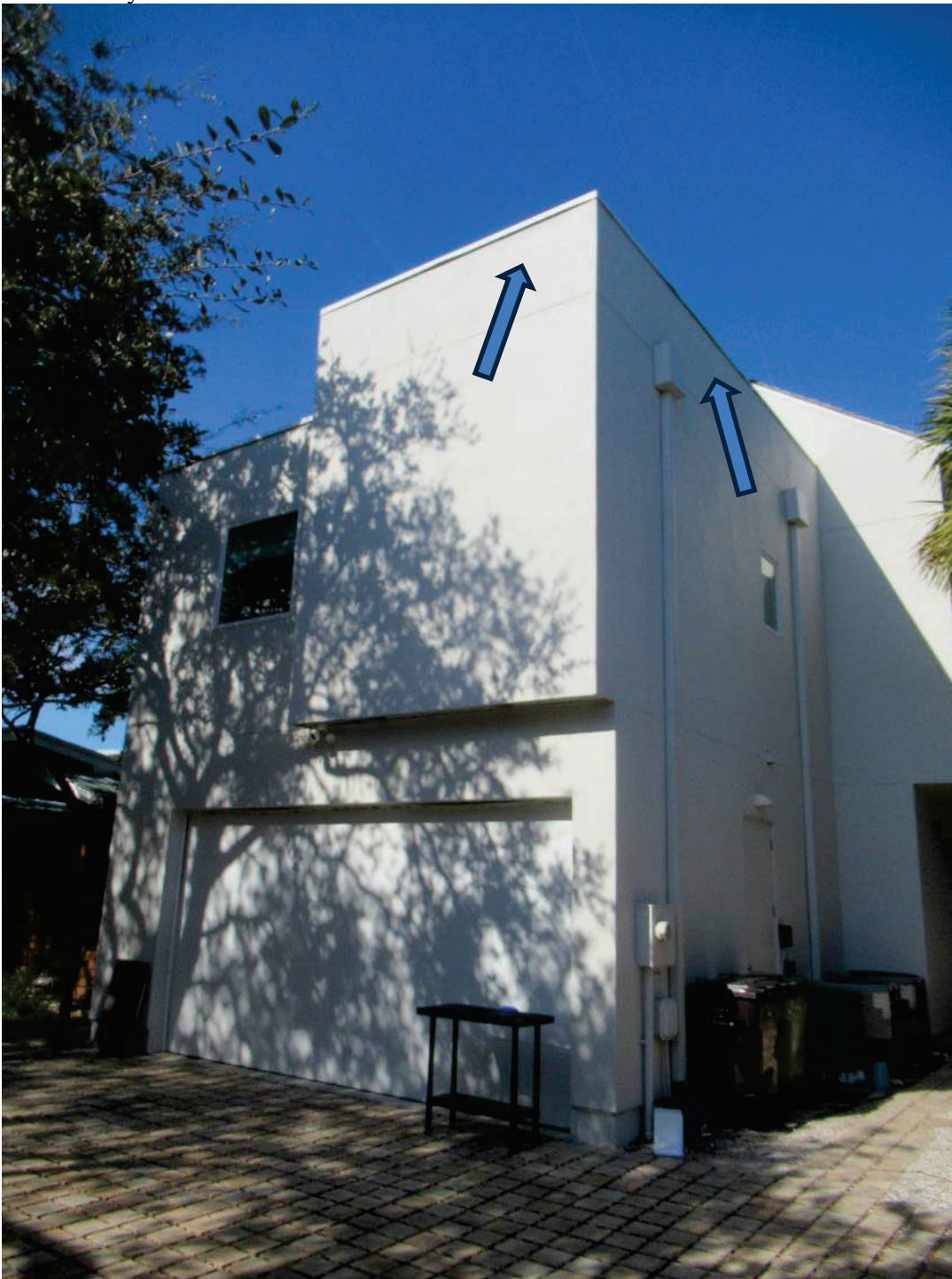
Photo of existing 3 rd story roof deck/roof garden with existing ½ wall at southeast corner. Existing half wall indicated by blue arrows.
