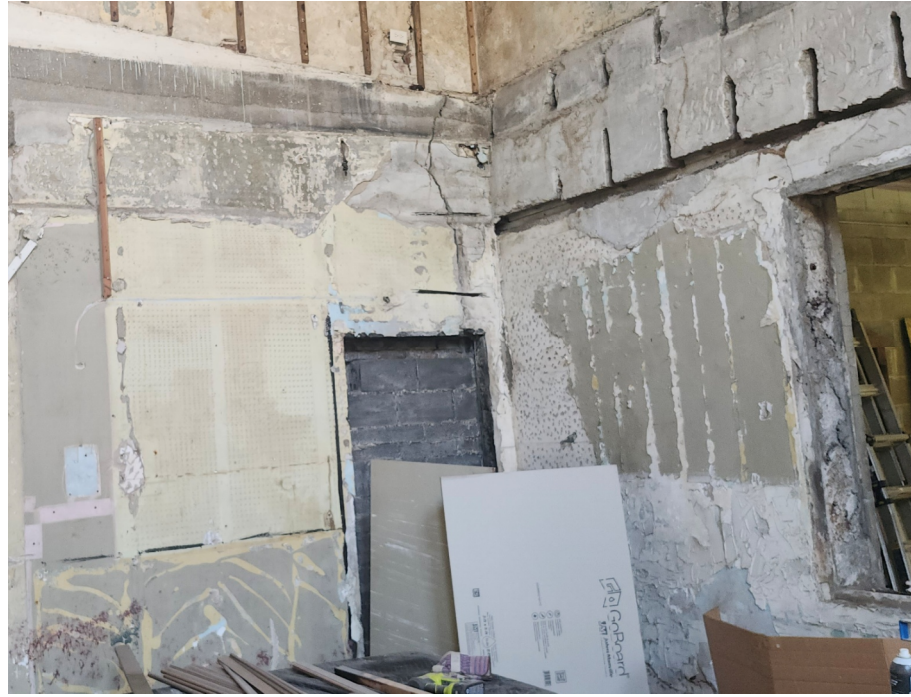
Photograph 3 - Cracked Coquina Wall
