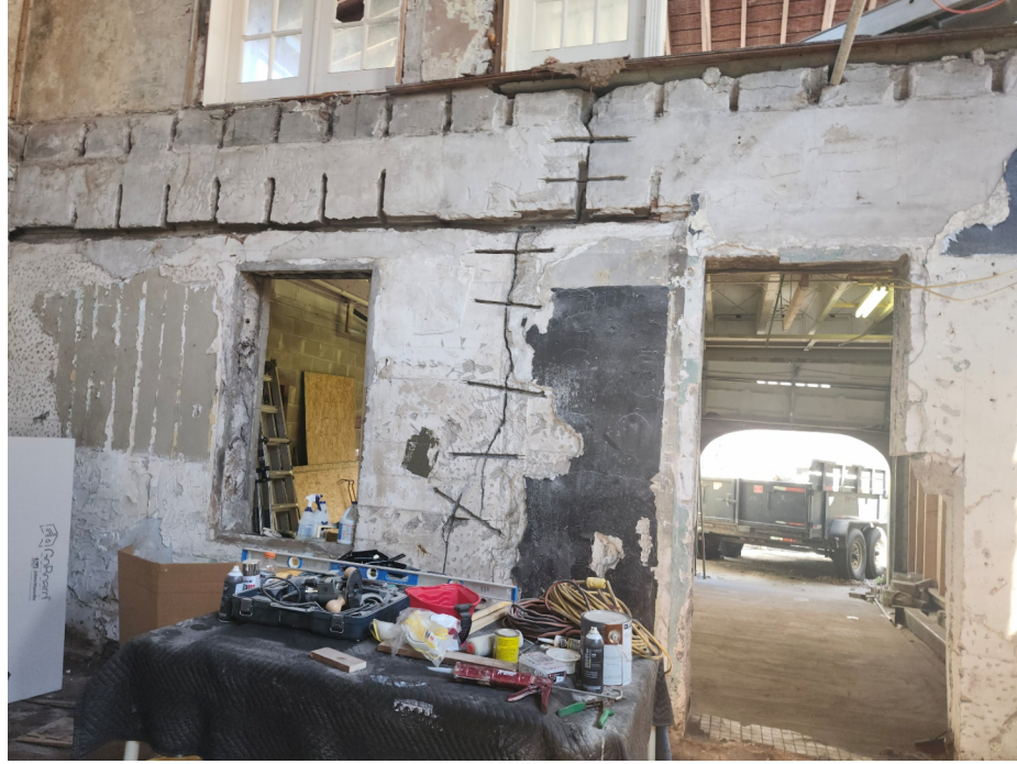
Photograph 1 - Cracked Coquina Wall
