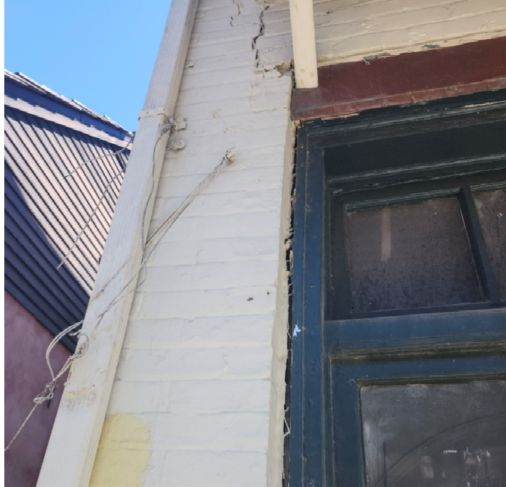
Photograph 9 - Brick Separating at Northwest Corner
