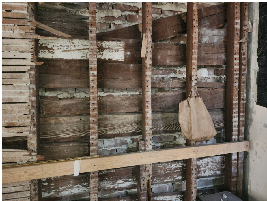
Photograph 8 - Deteriorated Brick Veneer and Stud Wall
