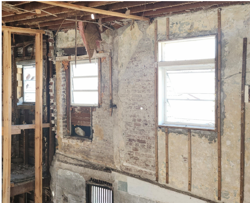
Photograph 6 - Damaged/Deteriorated Brick Wall
