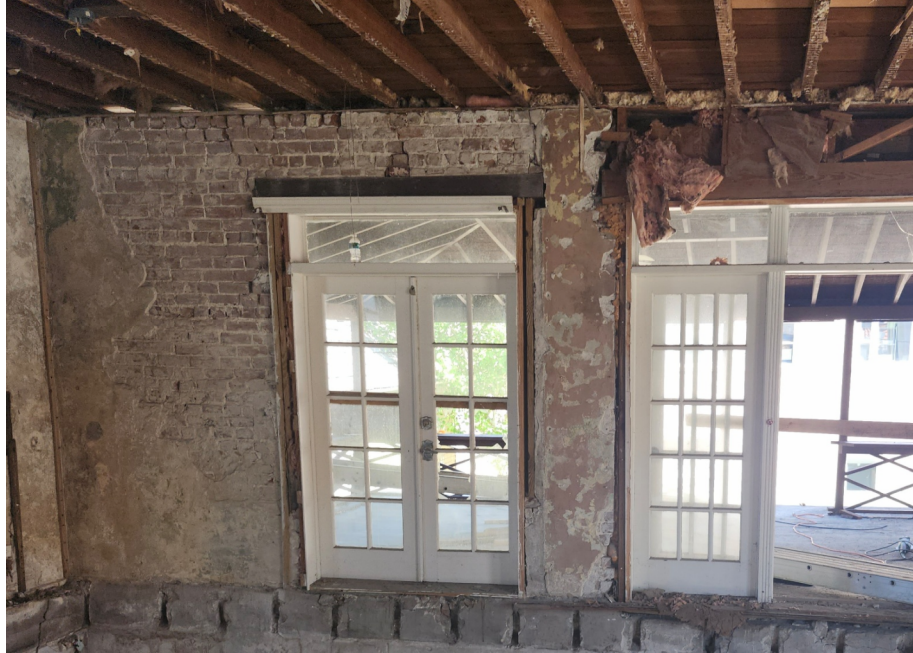
Photograph 5 - Damaged/Deteriorated Brick Wall
