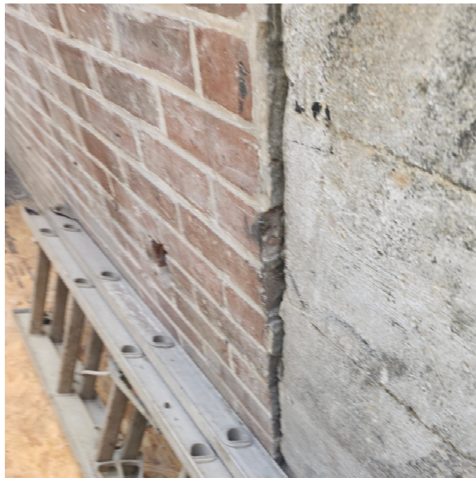
Photograph 10 - Brick Separating at South Wall
