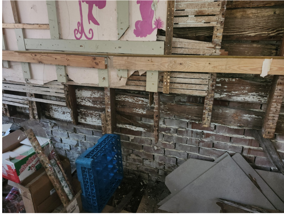
Photograph 7 - Deteriorated Brick Veneer and Stud Wall
