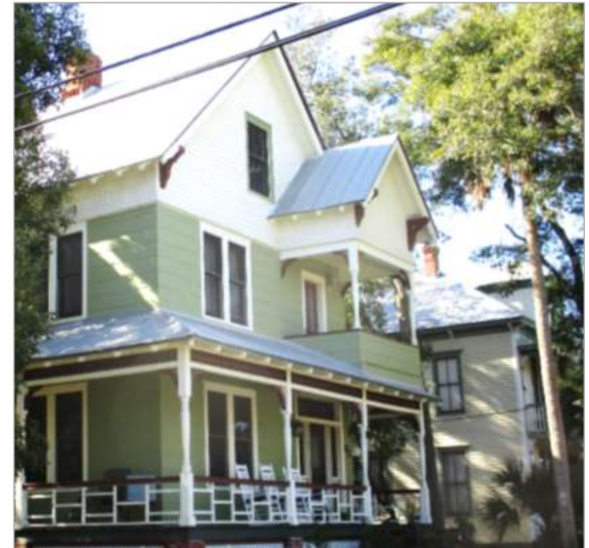
The siding on this building was altered (ca. 1930-50s) and shows the impact of replacement finishes that change the scale and detail of the building's historic character. Restoring the Queen Anne siding would be a staff-approvable request. Also note for reference the scale of historic horizontal siding shown on the adjacent historic building.
